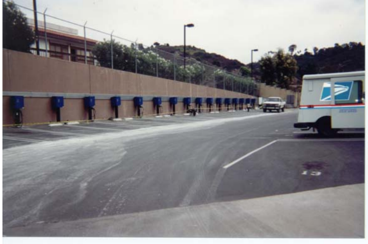
Figure 5-23. Example of a Level 2 commercial electric vehicle charger installation.
