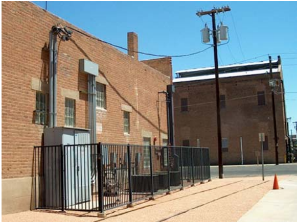
Figure 5-16. Typical commercial electrical supply panel.
