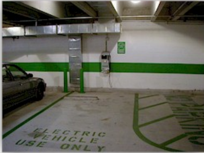
Figure 5-9. Example of ground striping for an Americans with Disabilities Act-compliant electric vehicle station.
