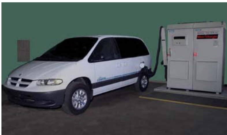
Figure 5-7. Level 3 fast charger (90 kW) for the Chrysler EPIC.
