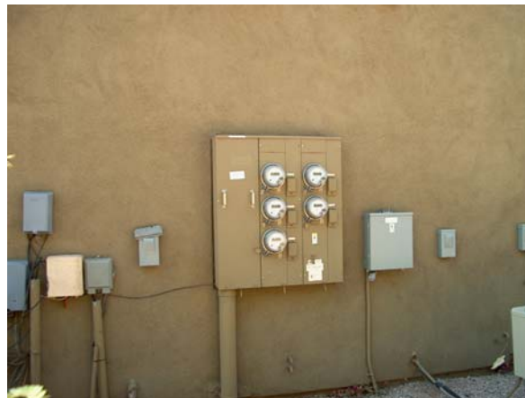
Figure 5-15. Typical apartment electrical distribution point.
